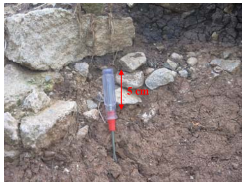
GAMBAR 10: Foundation rock of road at Barugbug sub village goes down approximately 5 cm because active fault influence (documentation: January 2005)
